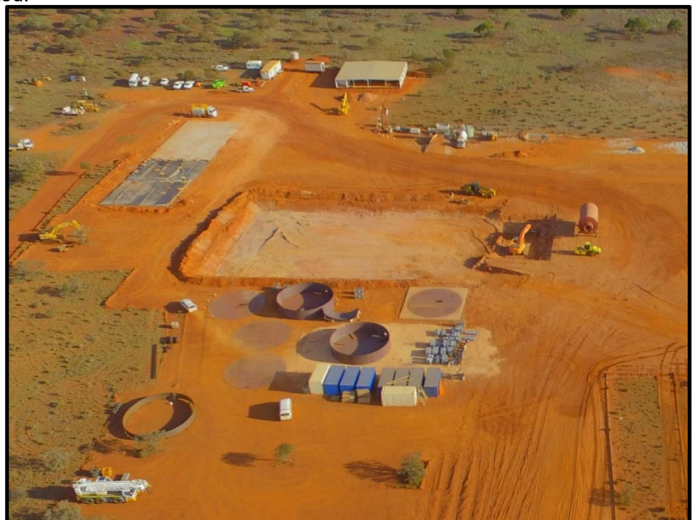
Figure 1: Aerial photo of the LGP Plant site showing administration block (top workshop concrete pad (far left) excavations for CIL tank farm (centre) and beginning of CIL tank construction (bottom)
